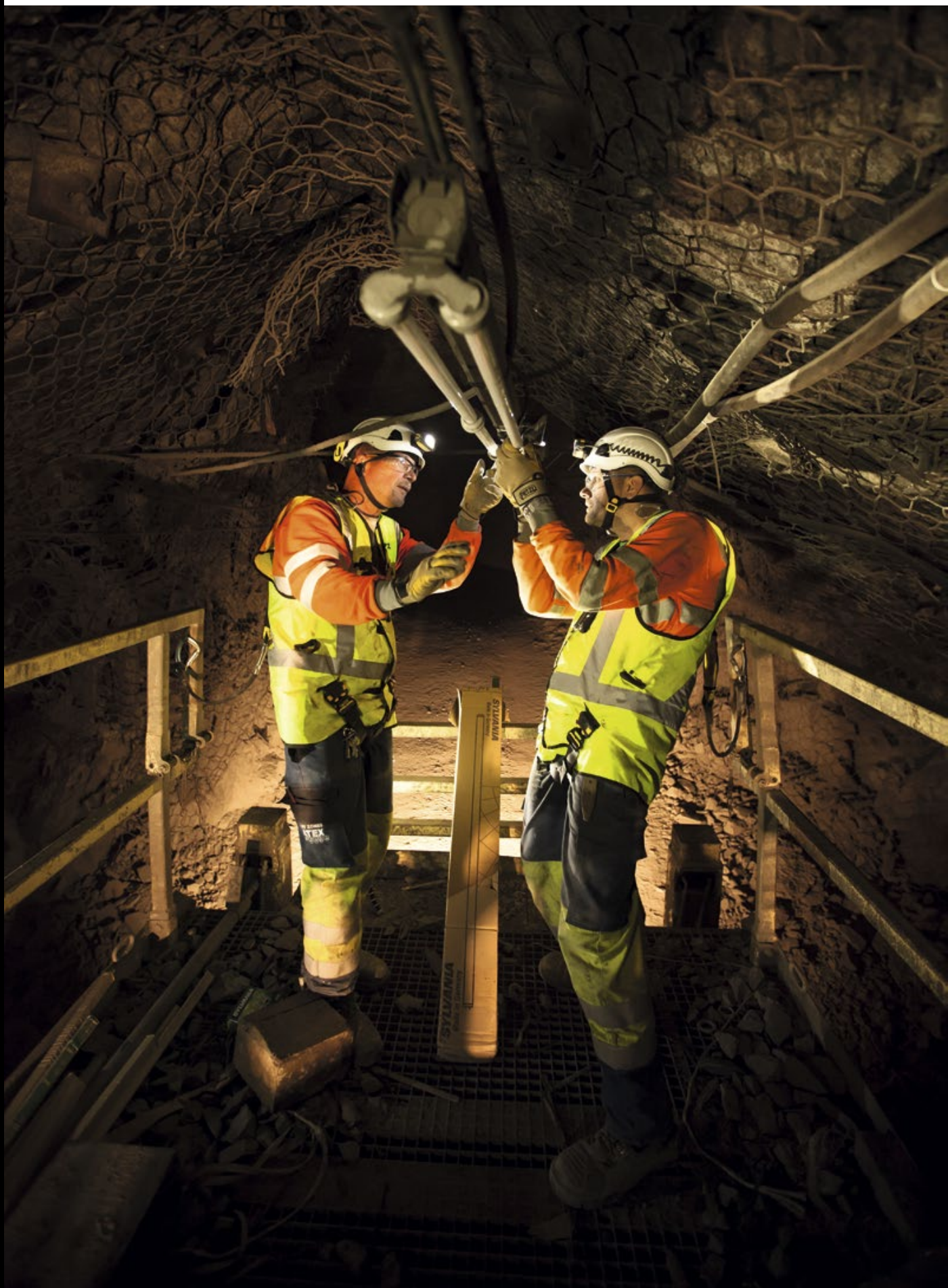
Replacement and maintenance of the lighting system inside a cement mine. France. © Petzl / Lafouche / Vicat
